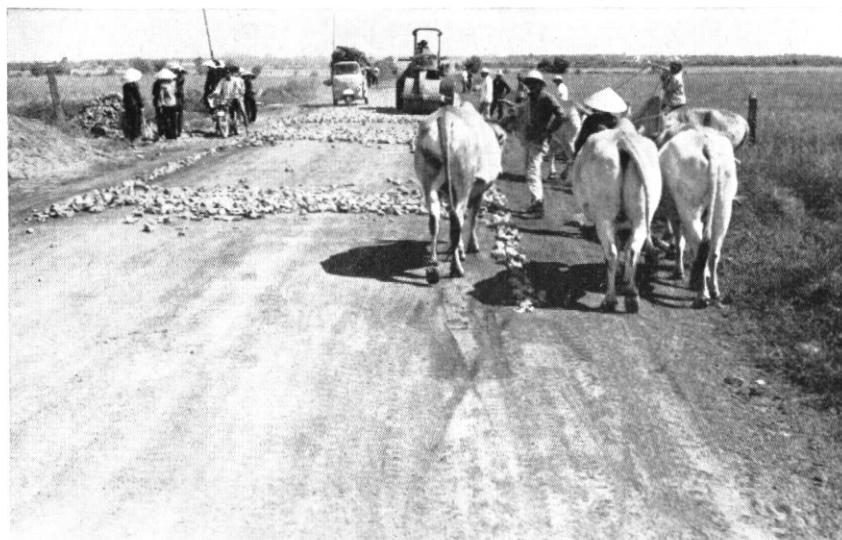
Provincial laterite road between Ba Ria and Hoa Long in Phuoc Tuy Province being prepared for sealing by Public Works Department.
